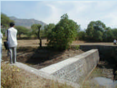
Many small structures in a catchment can add significantly to aquifer recharge. A recharge dam near Pune, India.
